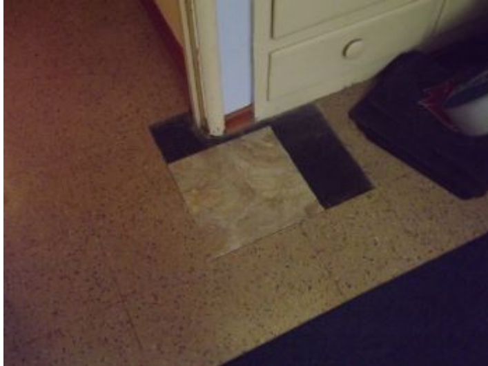
damaged 9X9 vinyl tile
