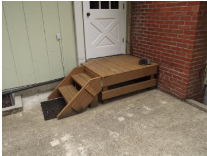
stairs without handrail
