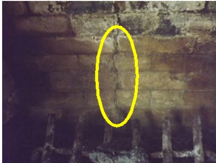
vertical crack in firebrick
