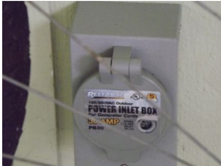
generator inlet plug
