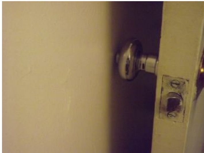
no doorstop will lead to wall damage
