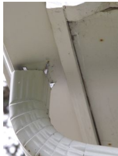
inadequately attached downspout
