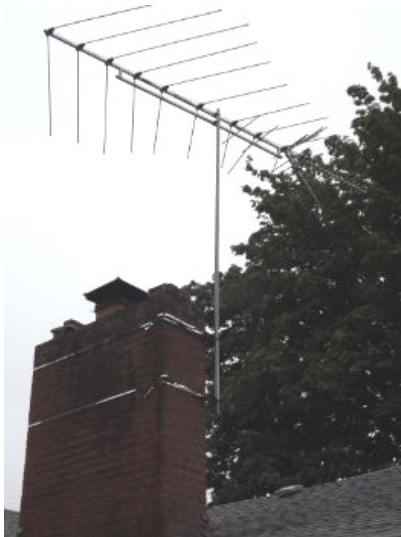
antenna attached to chimney
