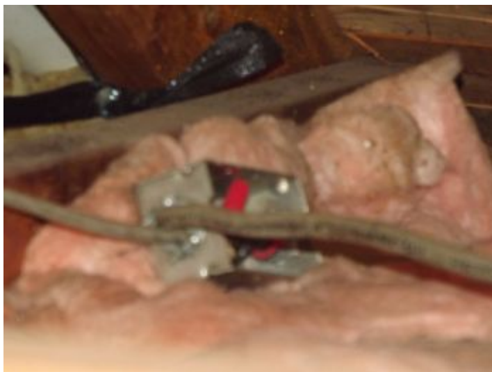
unsecured and uncovered electrical box
