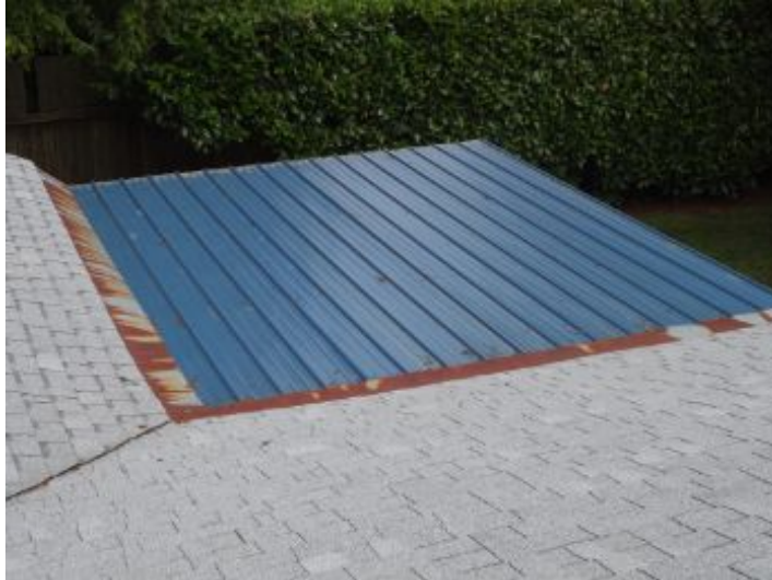
corroding transition sheetmetal
