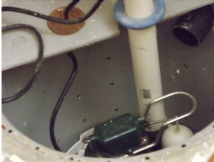
interior of dry sump pump
