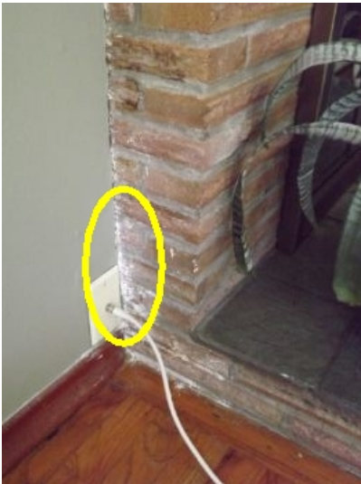
efflorescence at side of fireplace
