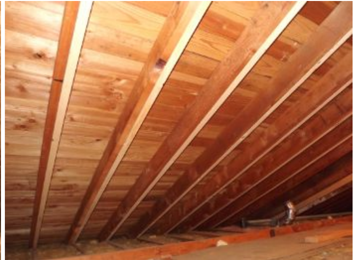
'sistered' roof rafters
