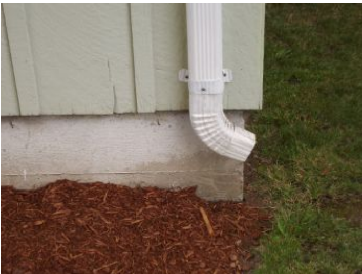
downspout with no splashblock
