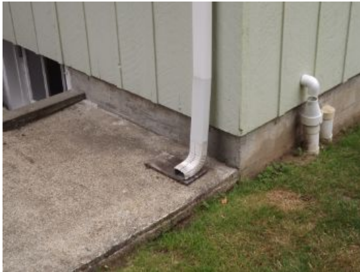
downspout without adequate splashblock
