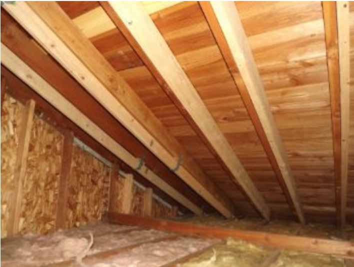
'sistered' roof rafters
