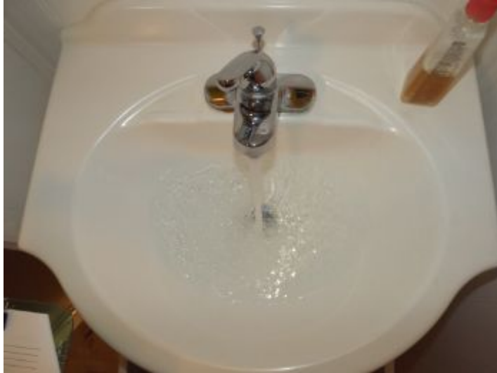
no overflow outlet in sink
