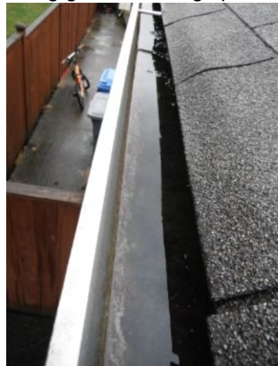
gutter full of water
