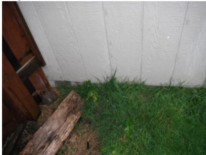
siding in close proximity to the ground
