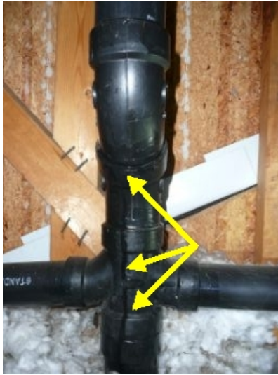
leaking plumbing vent line
