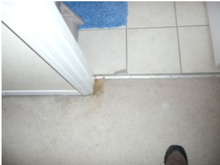
crack in floor
