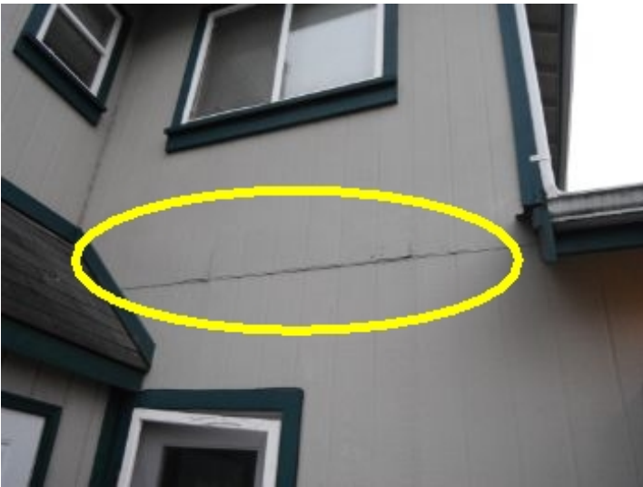
siding beginning to fail
