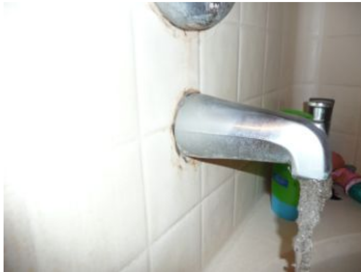
faucet in need of caulk
