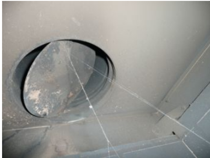
damper not fully closing
