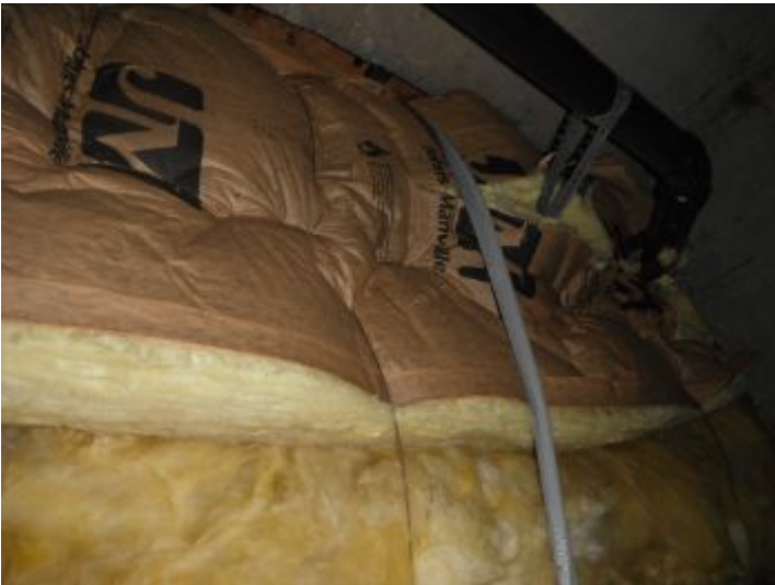
section of insulation installed upside down
