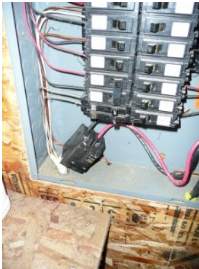
floating 50 amp breaker
