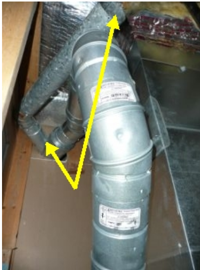
abandoned water heater vent
