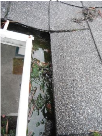
gutter full of water and debris
