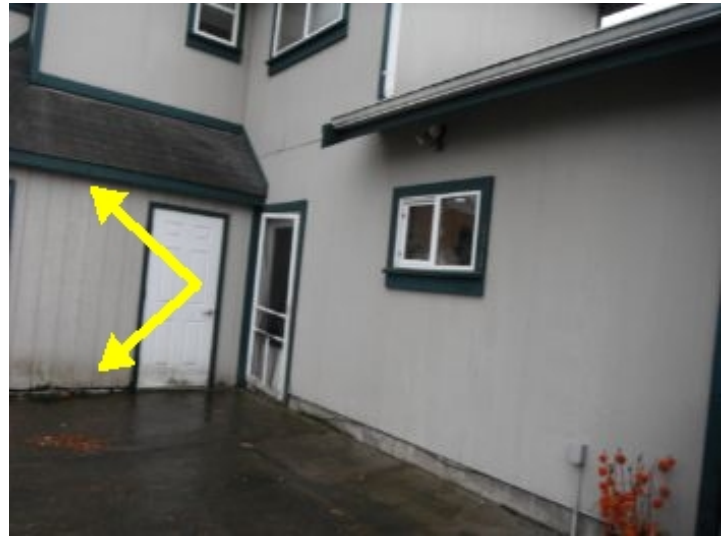
missing gutter causing splashing
